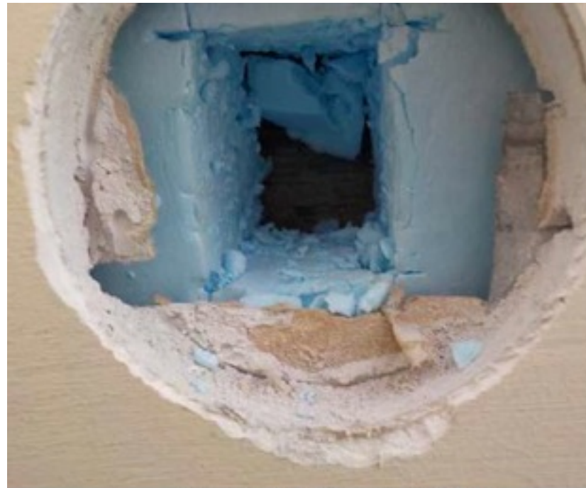
1450-Unit 211 - XPS rigid insulation
