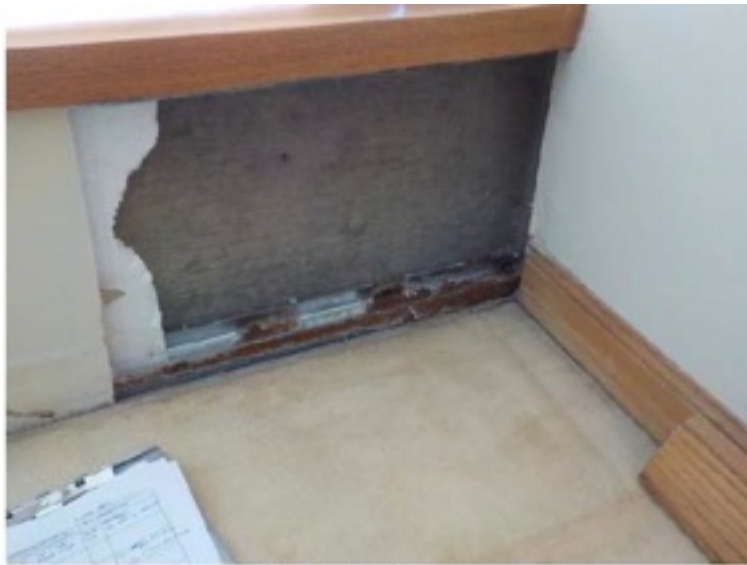
1450-Unit 211 - Corrosion on steel stud
