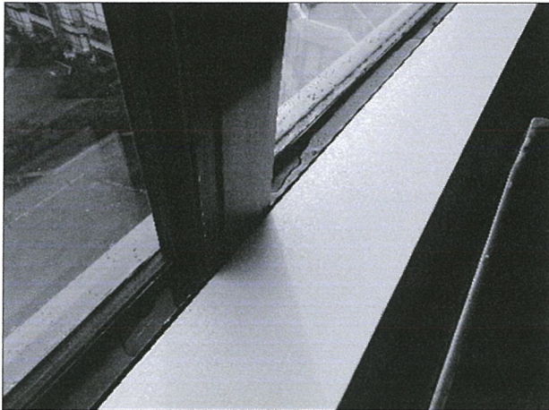
17 – Window leak in Unit 901 - 1470
