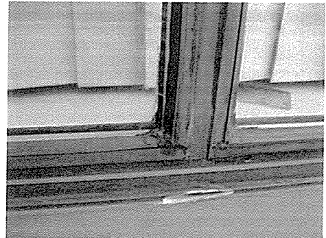
Photo 2: Glazing seals cut short and filled with failed sealant allows water to penetrate the window assembly.
