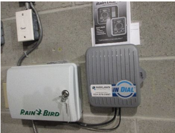
121 – Irrigation system controller
