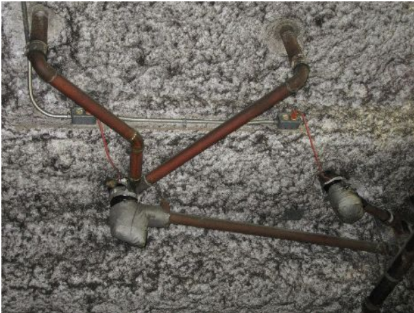
115 – Copper sanitary piping in parkade
