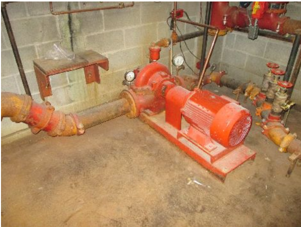
125 – Fire pump in 1450 water entry room
