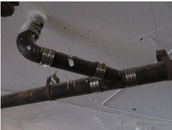
116 – Cast iron drainage piping in parkade
