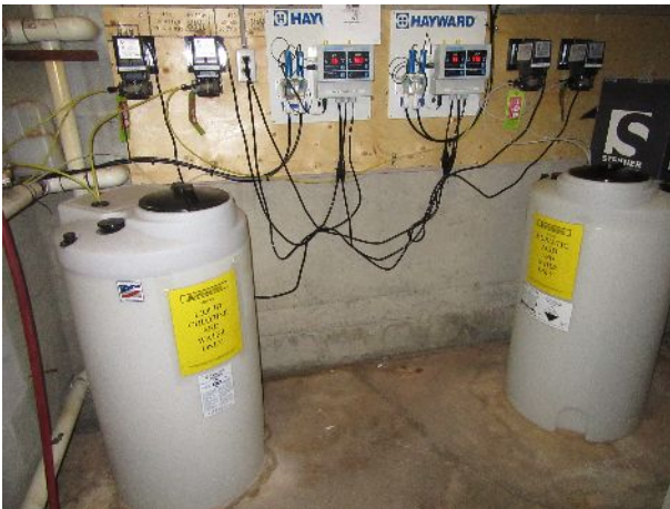
119 – Chlorine generation and pH control system
