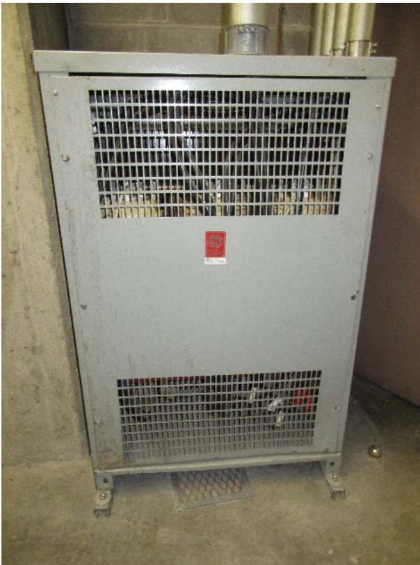
75 – Dry type transformer installed in electrical room
