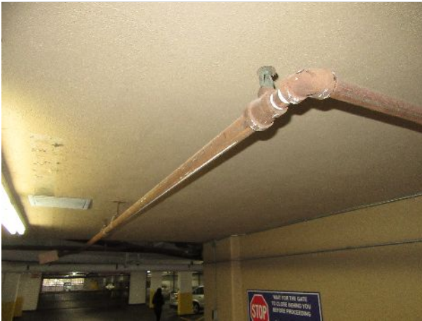
123 – Dry pipe sprinkler system piping and head
