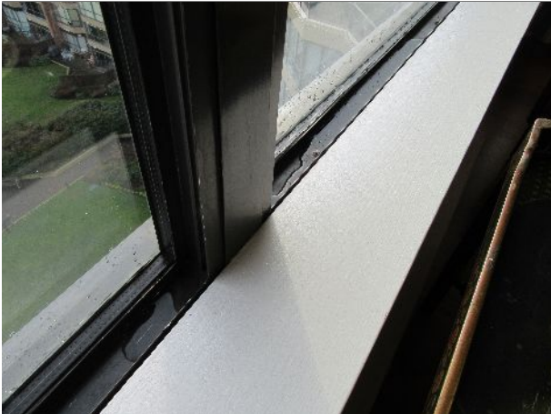
17 – Window leak in Unit 901 - 1470
