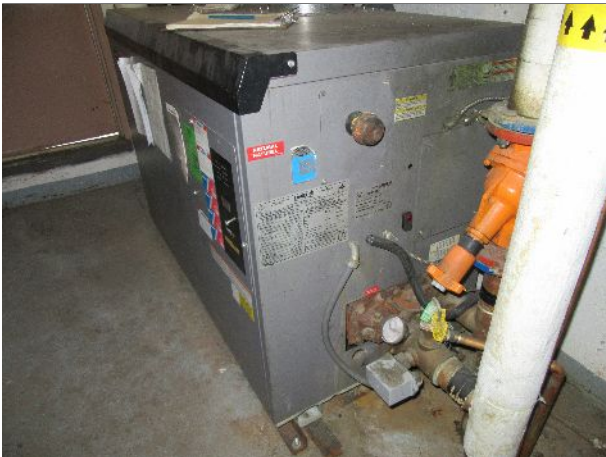
111 – Boiler in 1490 rooftop boiler room
