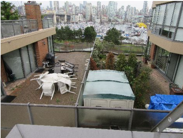
11 – Aluminum guardrails and privacy screens
