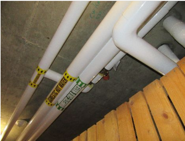
107 – Insulated copper piping in storage locker room
