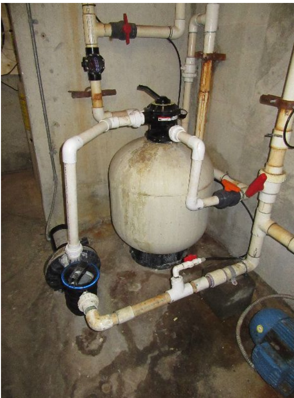
120 – Sand filter and pumps for hot tub
