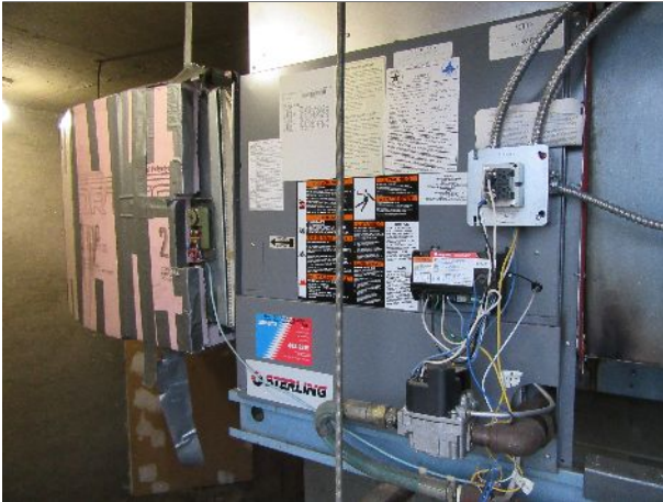
100 – 1490 AHU inside mechanical room
