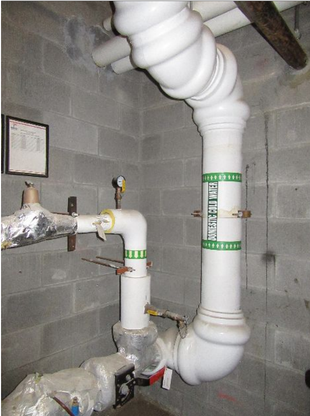
108 – Insulated copper piping in water entry room
