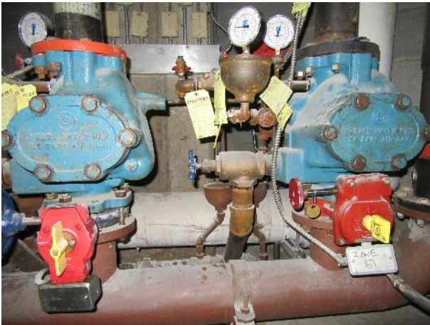
127 – Clapper valves in 1490 water entry room
