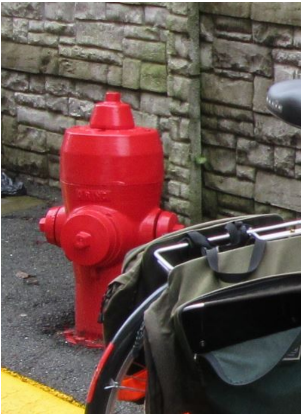
130 – Fire hydrant adjacent to Pennyfarthing Drive
