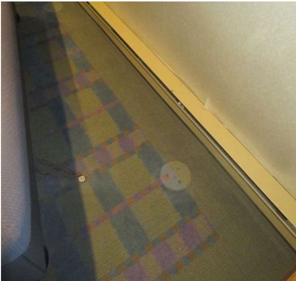
79 – Electric baseboard heater in entrance lobby
