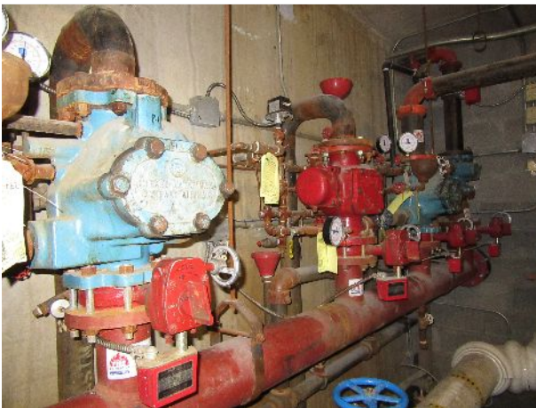
128 – Clapper valves in 1470 water entry room
