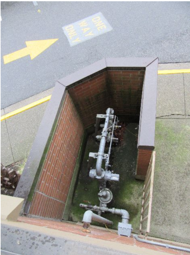
65 – Brick enclosure around gas meters
