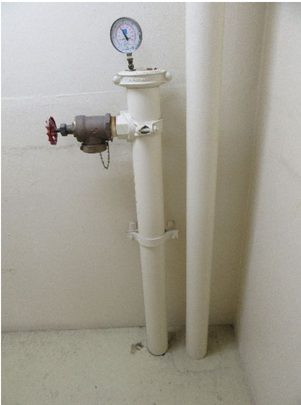
126 – Wet standpipe connection in stairwell
