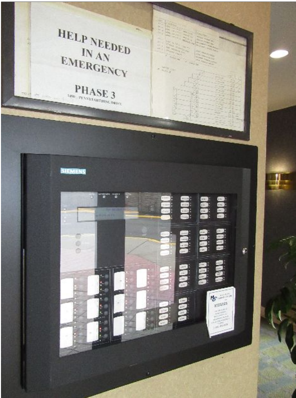
90 – Siemens annunciator panel in 1490 building
