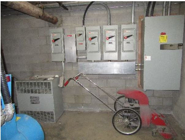
78 – Emergency power distribution equipment
