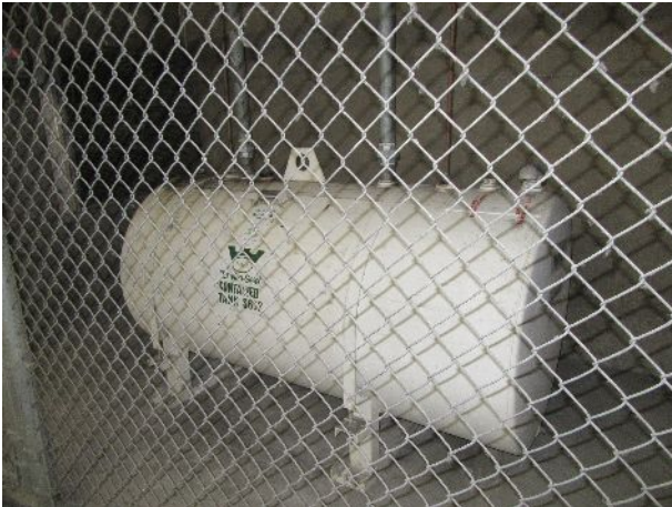
131 – Main fuel storage tank next to generator room
