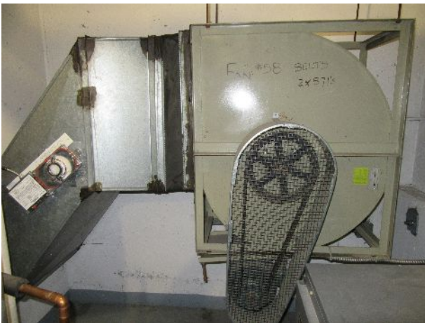
102 – Stairwell pressurization fan
