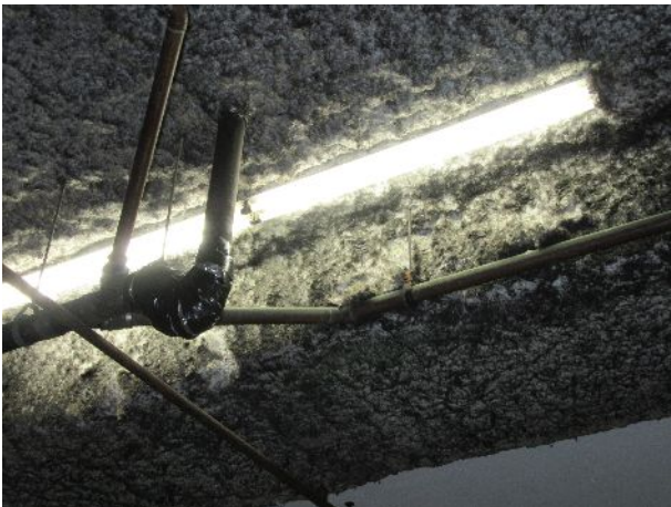
87 – T8 fluorescent strip light in parkade
