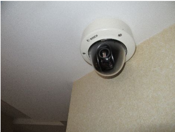
93 – Camera at 1470 entrance lobby
