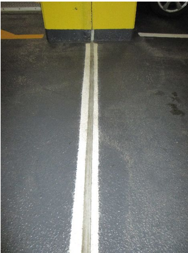
137 – Expansion joint in 1450 parkade
