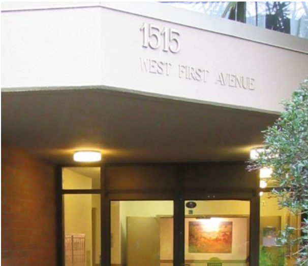
83 – Soffit-mounted entrance lights
