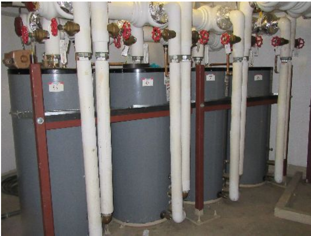
112 – Storage tanks in 1450 rooftop boiler room
