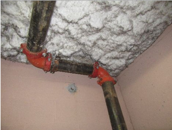
124 – Sprinkler piping in bicycle storage room
