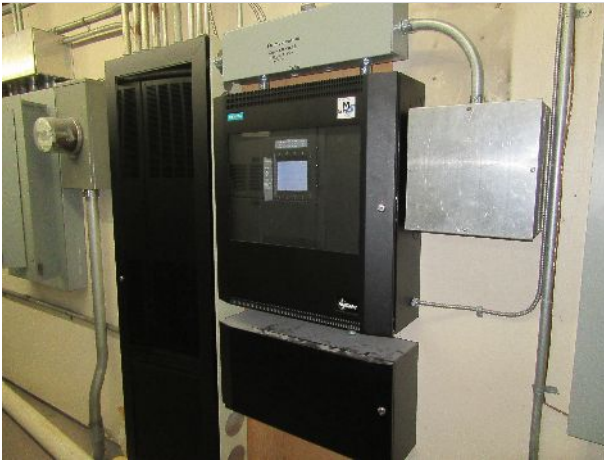
89 – Siemens FireFinder XLS fire alarm control panel
