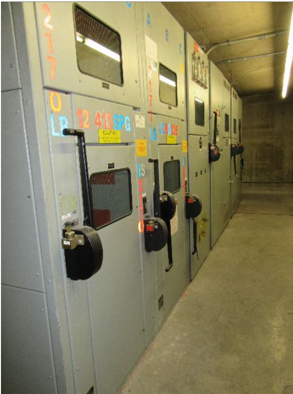
74 - Dual radial unit substation
