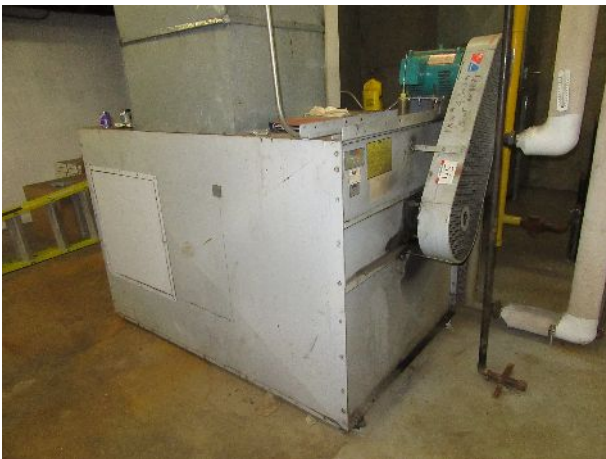
101 – Swimming area AHU
