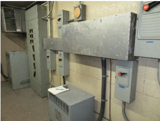
76 – Electrical equipment in 1490 electrical room
