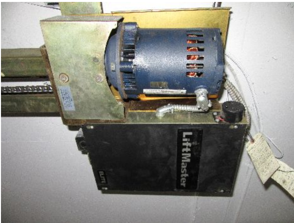
134 – Overhead gate operator
