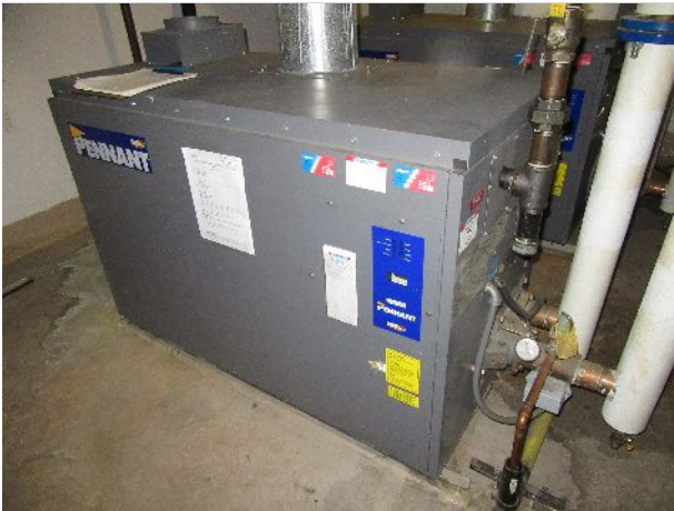
110 – Boiler in 1450 rooftop boiler room
