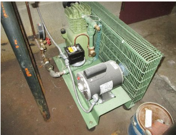
129 – Dry pipe sprinkler system air compressor in 1450
