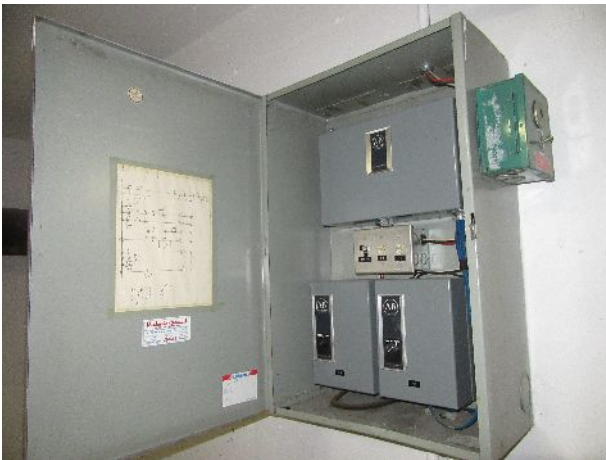
117 – Sump pump control panel
