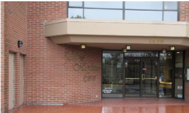
82 – Soffit and wall light fixtures
