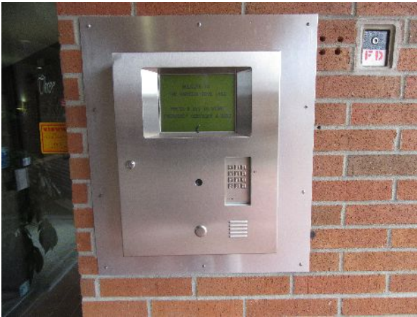
91 – 1490 telephone entry system panel
