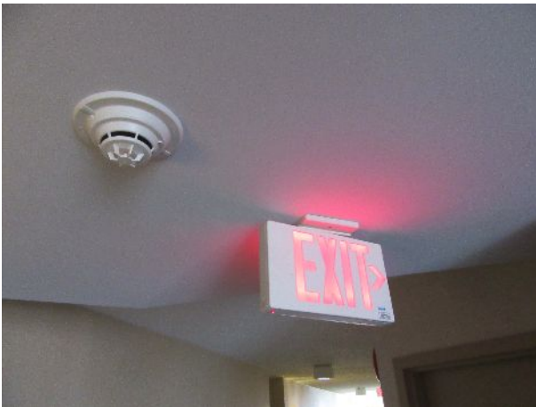
88 – Plastic emergency exit signage
